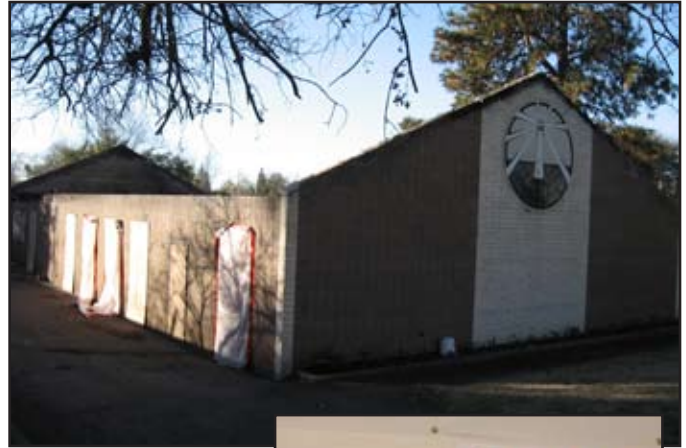
Above: Burned out shell of Grace Baptist Church
